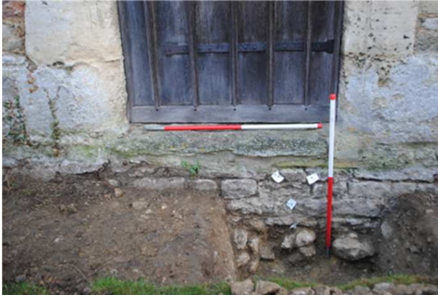
Figure 60 1m length of Structure [1048] off set to S (right) of Chapel W door. Upper 4+ dressed stone courses visible beneath the stone door step. The lower 2+ rough cut courses are set into clay.
