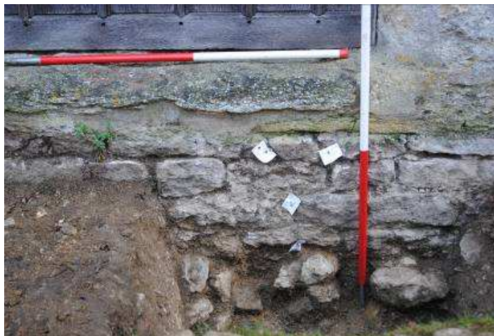
Figure 59 The line of large rough stones revealed (bottom of photo) over the clay base of 1m slot seems to indicate an earlier phase under the previously revealed three courses of dressed stonework beneath the existing chapel W door.
