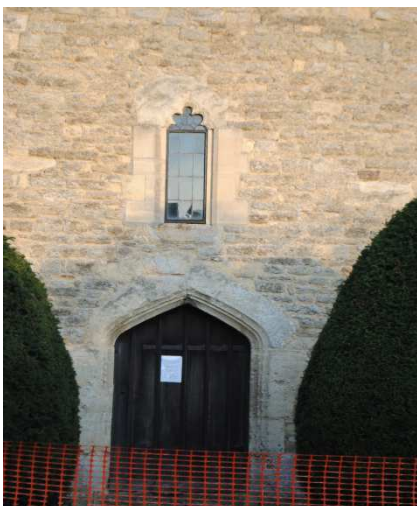
Figure 61 W wall of existing chapel showing W doorway with moulded jambs and segmental pointed head thought to be late 14 th century? But why is there clear evidence above its head (to N/left) of half the remains of an earlier segmental arch?
