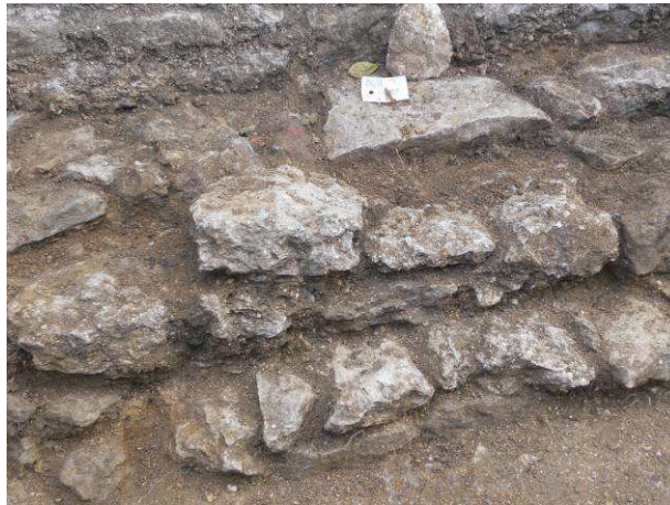
Figure 5 North-facing section showing the phases of [1036]: Phase 1 (lowest), 2 courses; Phase 2 (middle), 2 courses; Phase 3 (upper, slightly recessed), one course of larger flags.
