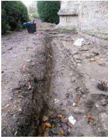
Figure 32 Looking E towards NE buttress, the north-facing edge of the stone courses of [1037] can be clearly seen. See also above Fig. 26 (looking W) and Fig. 25 (footings). The substantial jutting 'footings' are visible to E before [1037] is seen to run under [1044]; also the section of the top course of [1037] missing/ removed further to W, with lower courses revealed (bottom right hand corner) as [1037] continues W.
