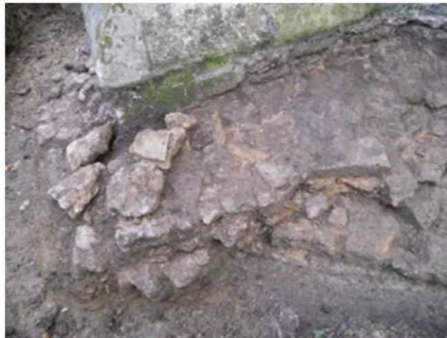
Figure 33 Stone courses of [1037] are seen to run under more substantial flags of [1044] which in turn run under NE buttress.
