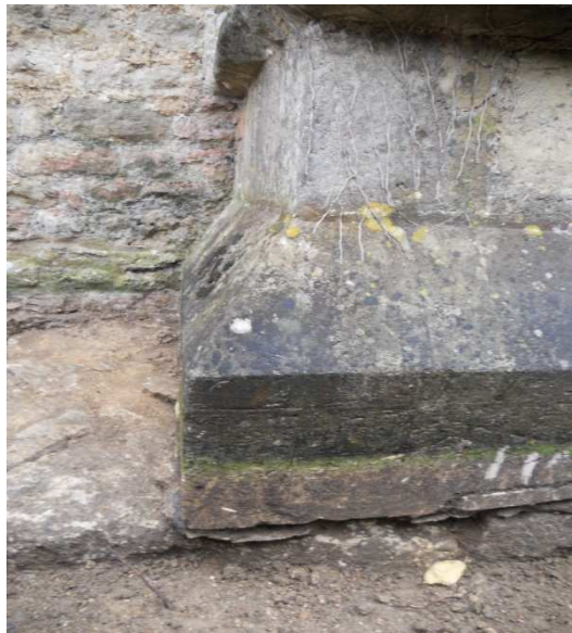
Figure 37 Large flagstone of [1045] runs W under two-thirds the width of N buttress. The buttress overhangs [1045] to N by 0.07m. It has been packed out to W of buttress to form a base for the later built buttress.
